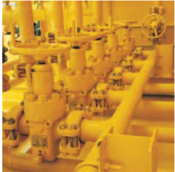
The use of Grayloc connectors, on a Centex Oil and Gas, Inc. platform in the Gulf of Mexico, saved 15" of horizontal space on the separator manifold of this skid-mounted production unit, and reduced the total topside platform weight by more than 11 tons.
